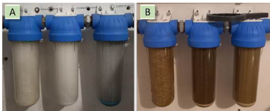
Figure 10. Whole-house filtration system consisting of 3 filters (filters from left to right: yarn, spun, carbon): A – clean filters immediately after installation, B – dirty filters requiring replacement
