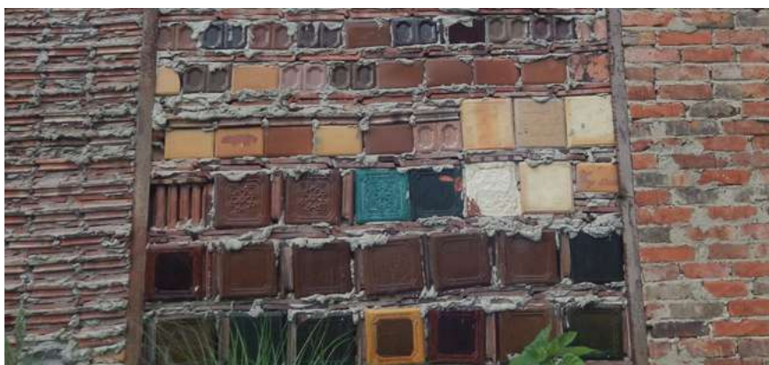
Photo 12.6. Tiles from Łązek Garncarski. View from the courtyard of Kasina Zagroda. Photo by Anna Mazurek-Kusiak
