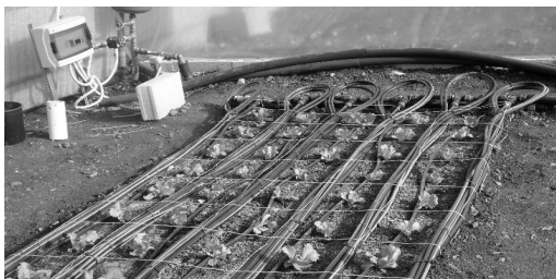
Figure 3. Heating system inside the greenhouse.
