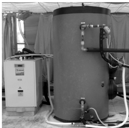
Figure 2. Heat pump and boiler.
